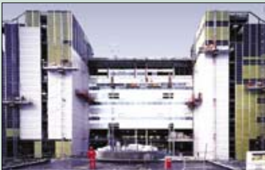
An example of a KTP project: Mastclimbing working platform, by Mastclimbers Ltd, in use at Atalantic Quay.
